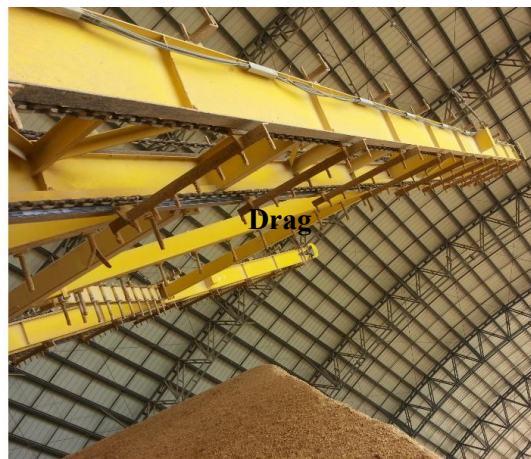
Figure 1. Drag system in the limestone reclaimer
