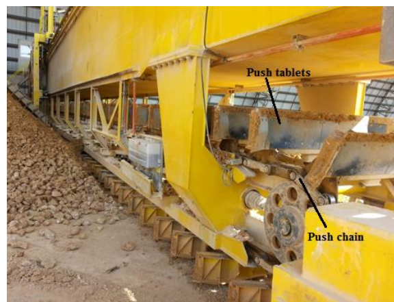
Figure 2. Push device in the limestone reclaimer.
