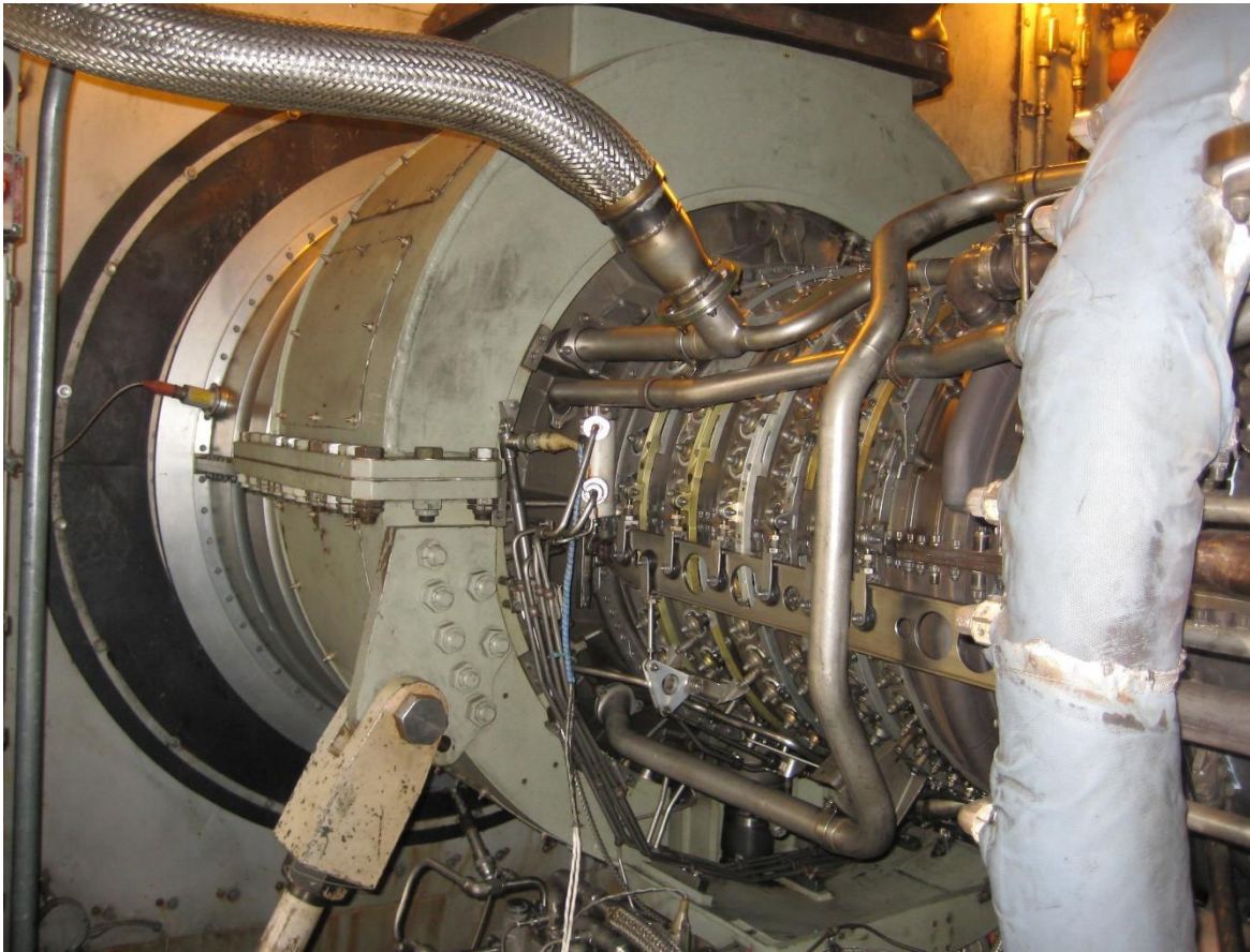
Figura I-1 Turbina a gas General Electric LM5000
