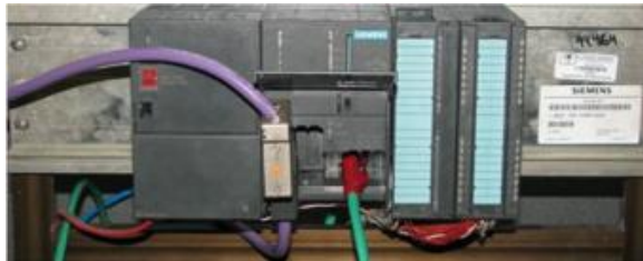
Figura 3. PLC S7300 Siemens CPU 315F 2PN/DP
