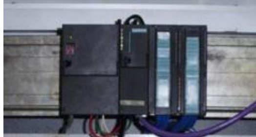
Figura 4. PLC S7300 Siemens CPU 314C 2DP
