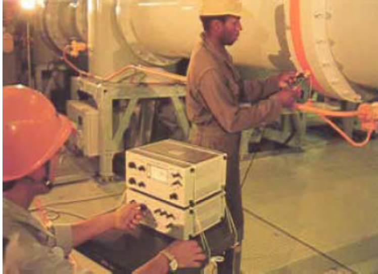
Tomada de 800 kV Gas Insulated Switchgear TOSHIBA*
