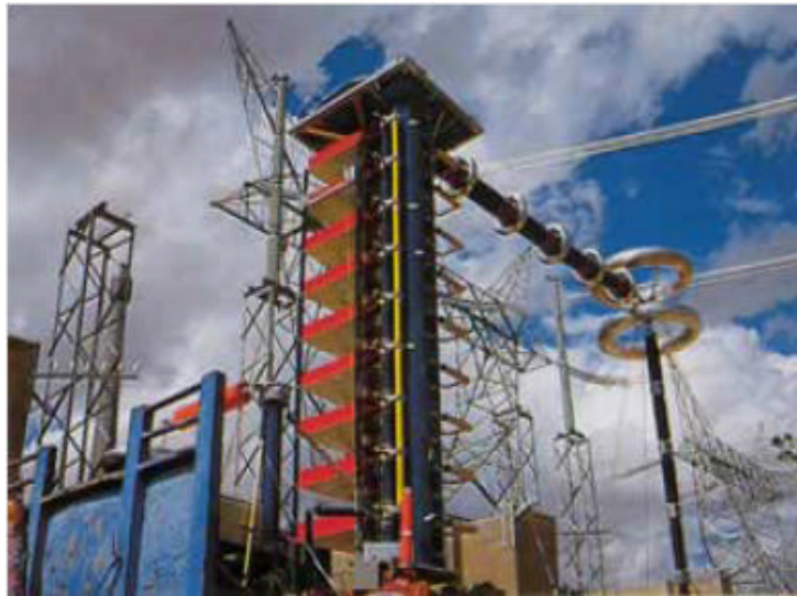
Tomada de 800 kV Gas Insulated Switchgear TOSHIBA
