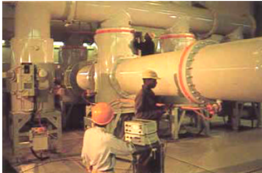
Tomada de 800 kV Gas Insulated Switchgear TOSHIBA
