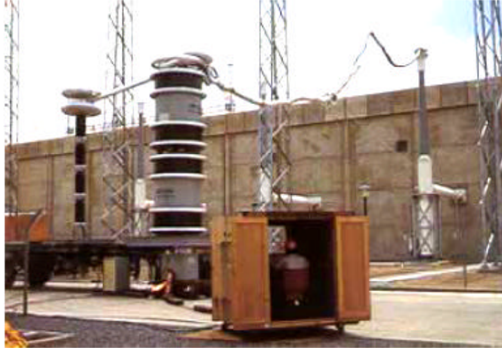
Tomada de 800 kV Gas Insulated Switchgear TOSHIBA*
