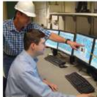
Central control room.
