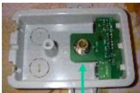
Figura 25a. Lightning Arrestor cable UTP
